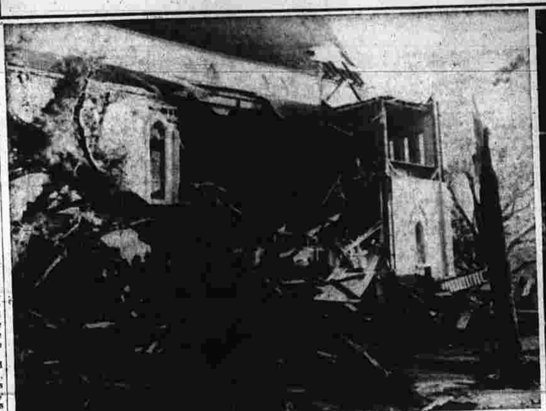
St. James Church had this gaping hole knocked in its side when the 1200-pound lead dropped through it during the height of the storm.
